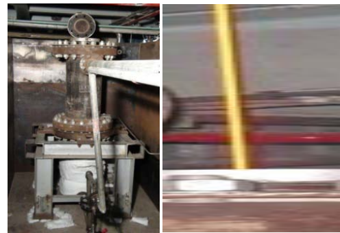
Fig. 19 (b): Picture of Test Facility
