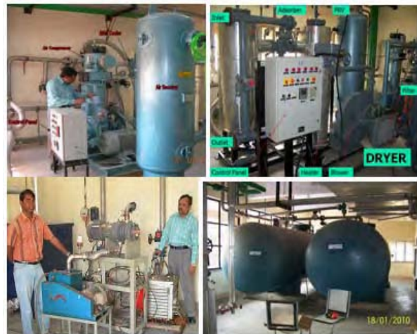
Fig.10: SF 6 Gas Transfer System.
